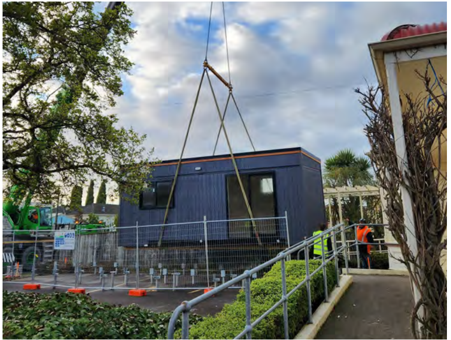
One of two new pods being craned onto the Knight Street site.
